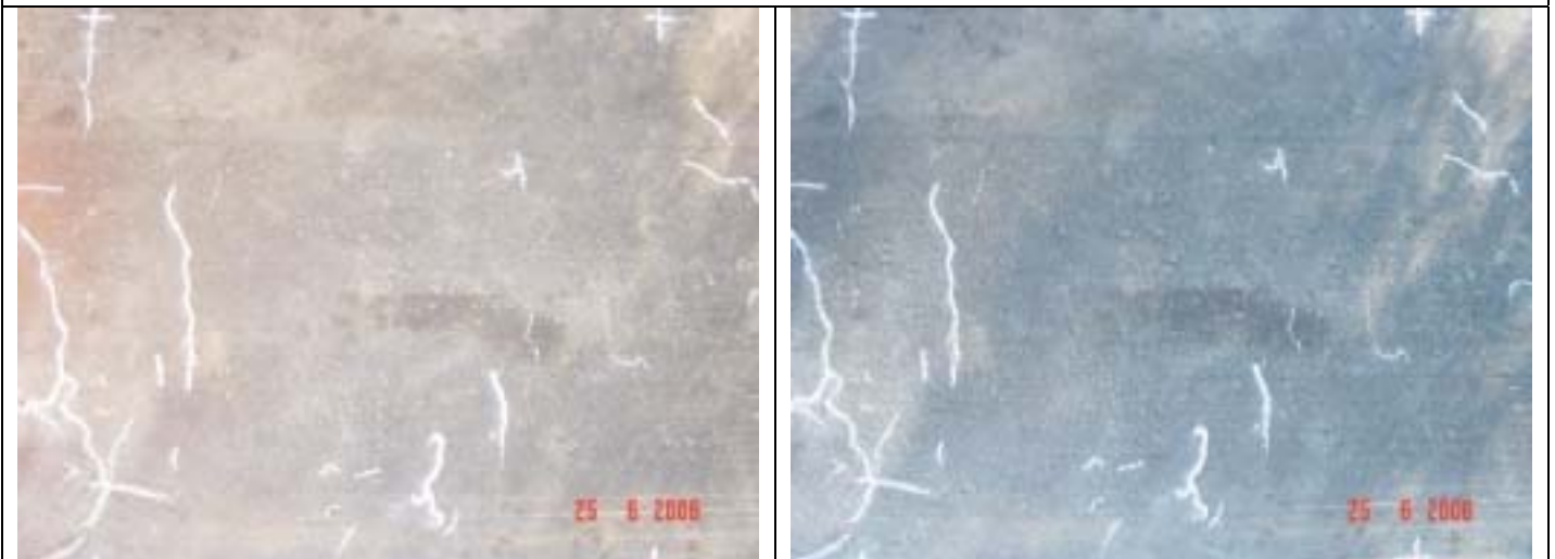
Plan views of test section with crack patterns marked with chalk
