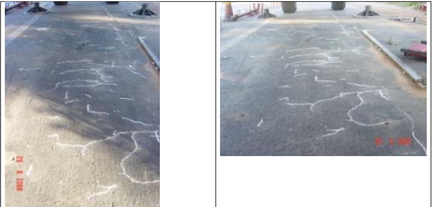
Pictorial overview of test section with crack patterns marked with chalk.
