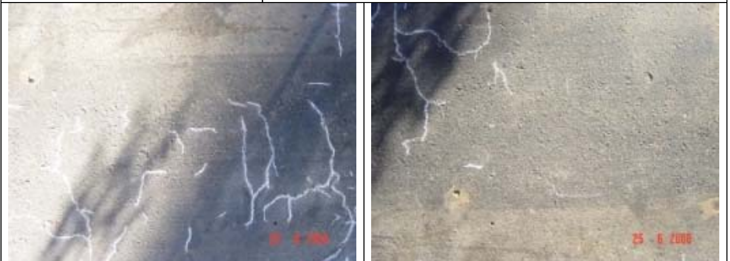
Plan views of test section with crack patterns marked with chalk
