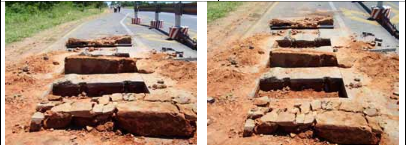
After completion of diagnostic trenching note reconstituted CTB slab in front of picture.
