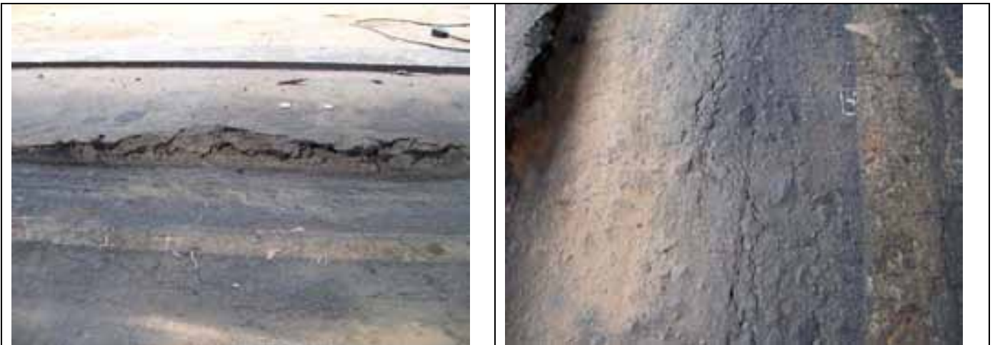
Heaved HMA on side of wheeltrack
