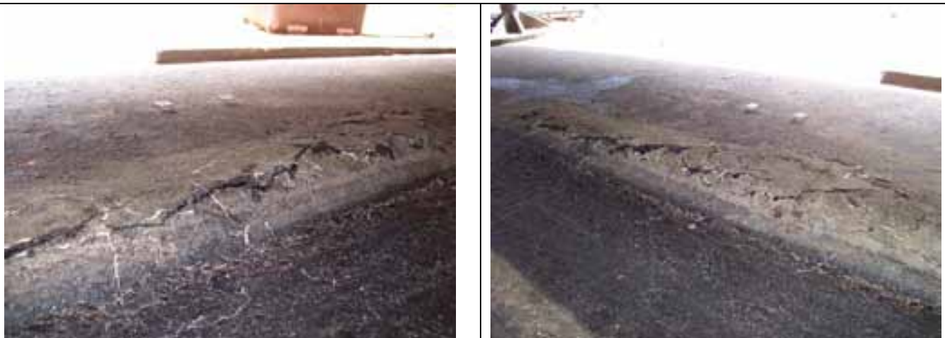
Vertical shear and disintegration on the sides of the wheeltrack
