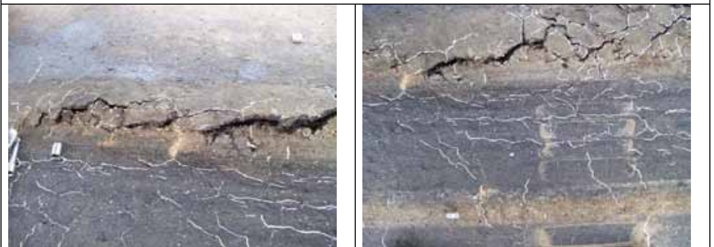
HMA heaving and cracking on the side of the wheeltrack. Note extensive crack pattern in wheeltrack
