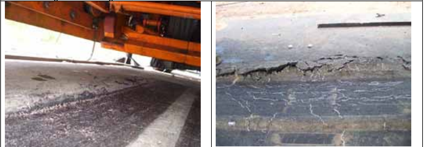
HMA heaving and cracking on the side of the wheeltrack
