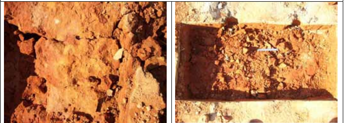
Fractured CTB and plan view of test pit after removal of CTB fractures.
