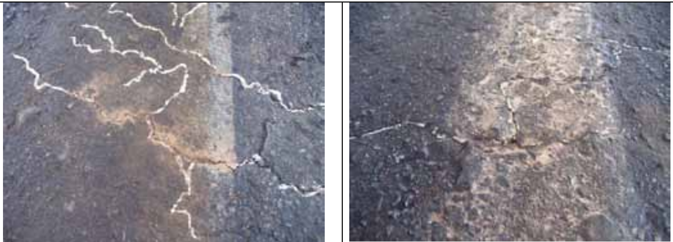
Close ups of material pumping through cracks in asphalt
