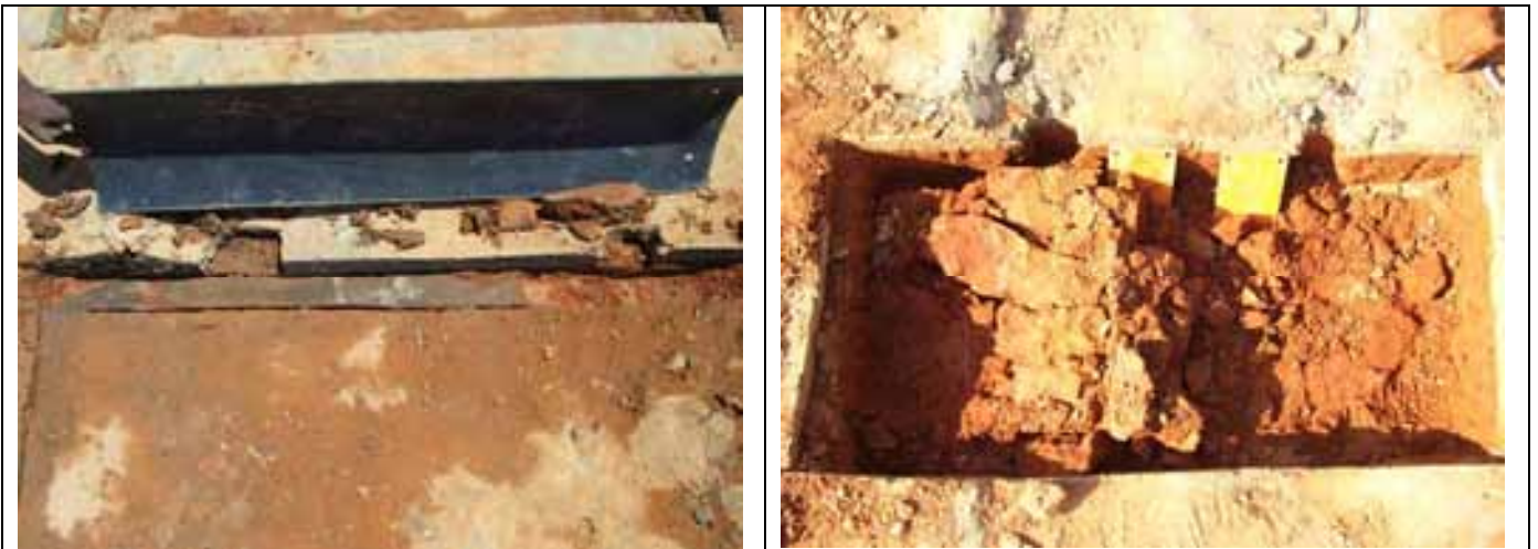
Removal of CTB fractures. Plan view of test pit during removal of CTB fractures note the size of the fractures.
