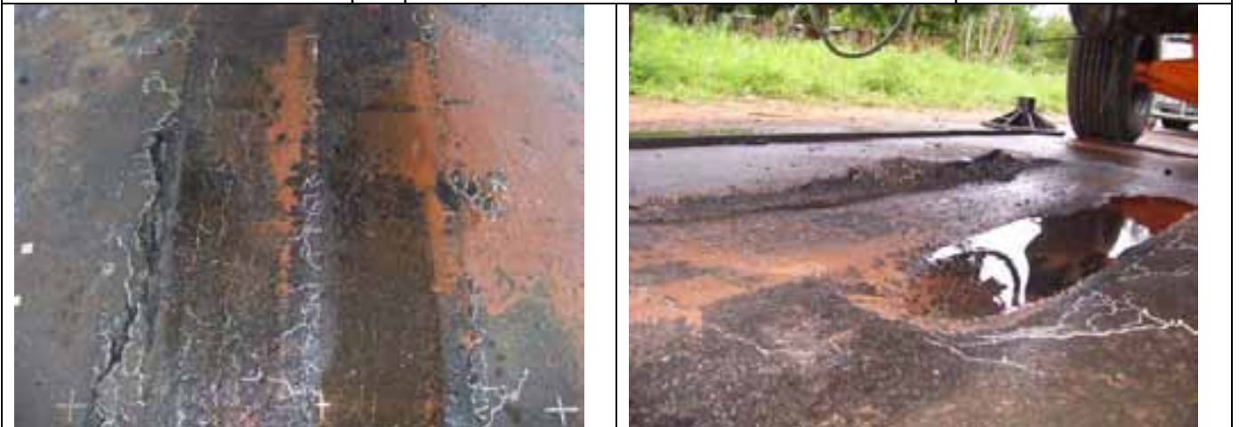
Plan and pictorial views of base material pumped out of test section. Note extensive crack patterns
