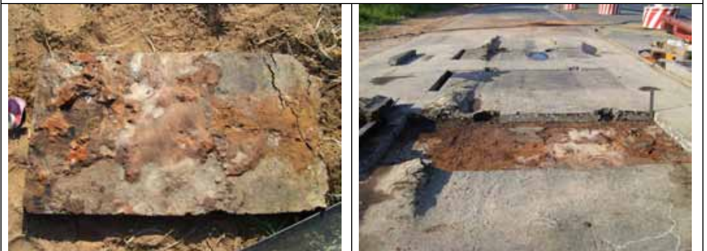
Underside of removed HMA mat. Note smoothed interface surface due to shear fatigue.
